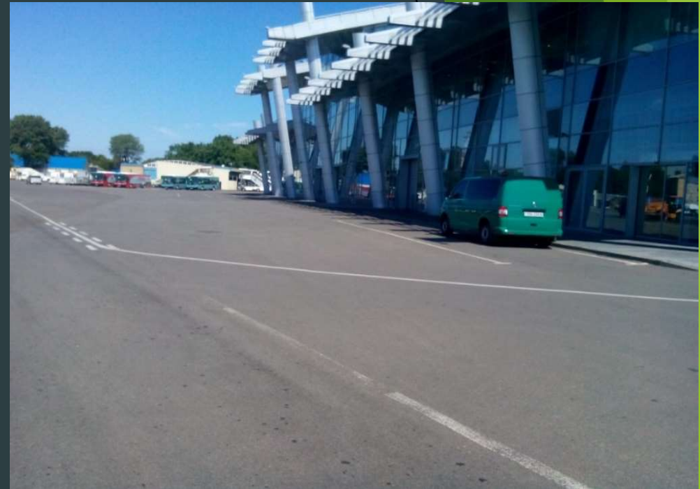
Repair works on taxiways in the aircraft parking area and car parks
